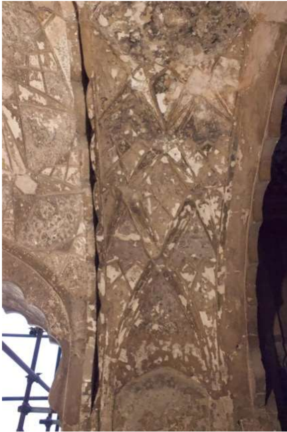
Figure 36 Archway DKKOA. Blackened paint.
